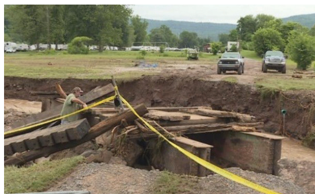
Washed out bridge in Summers Co. Mark Hughes, WVVA News Photographer
